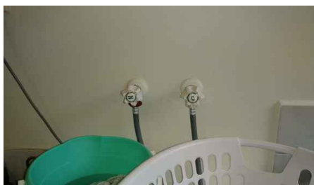
Washer Hook-ups: In serviceable condition at the time of inspection
